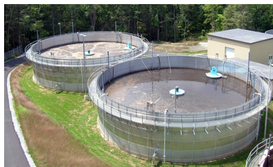
Figure 3: Sequencing Batch Reactors (Aqua-Aerobic Systems, Inc.)
