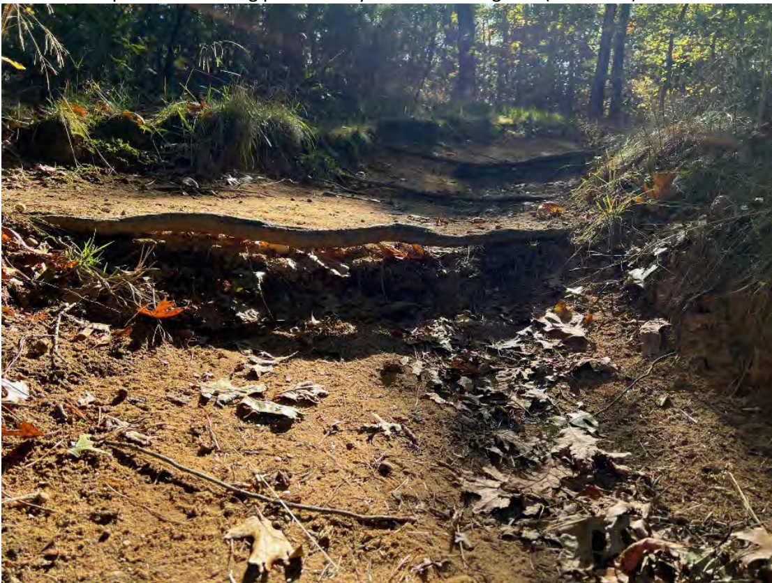
Photo 41: Representative exposed root systems/tripping hazard within trail (Cove Trail).
