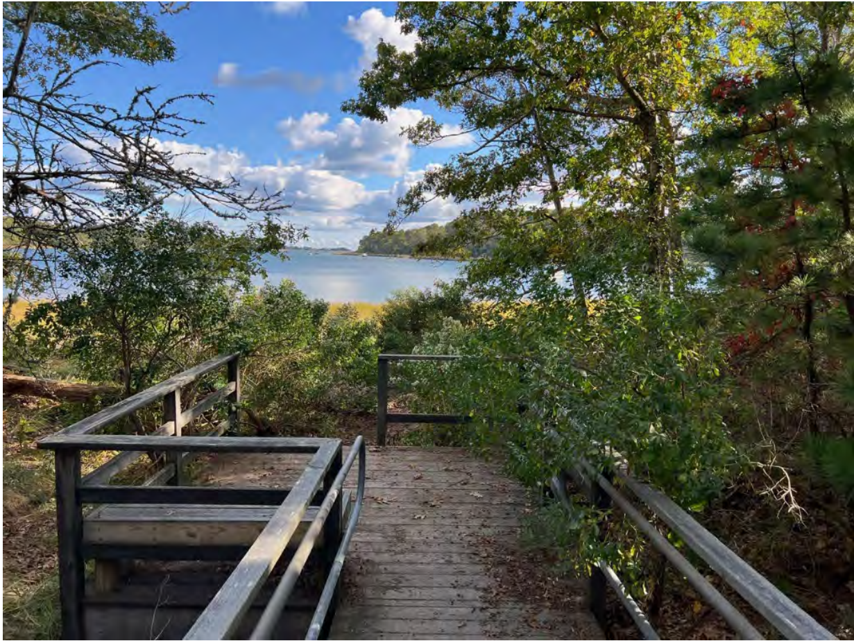
Photo 44: Ramp/boardwalk with encroaching vegetation.
