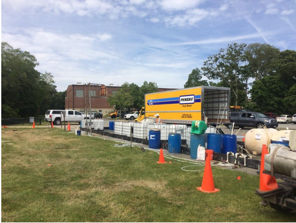
EVO totes in white. Injections into one direct- push point is in progress.
