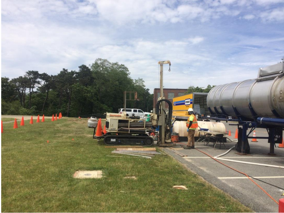
Injection area is blocked off by cones. The water tank is on the right and the drill rig in the center.
