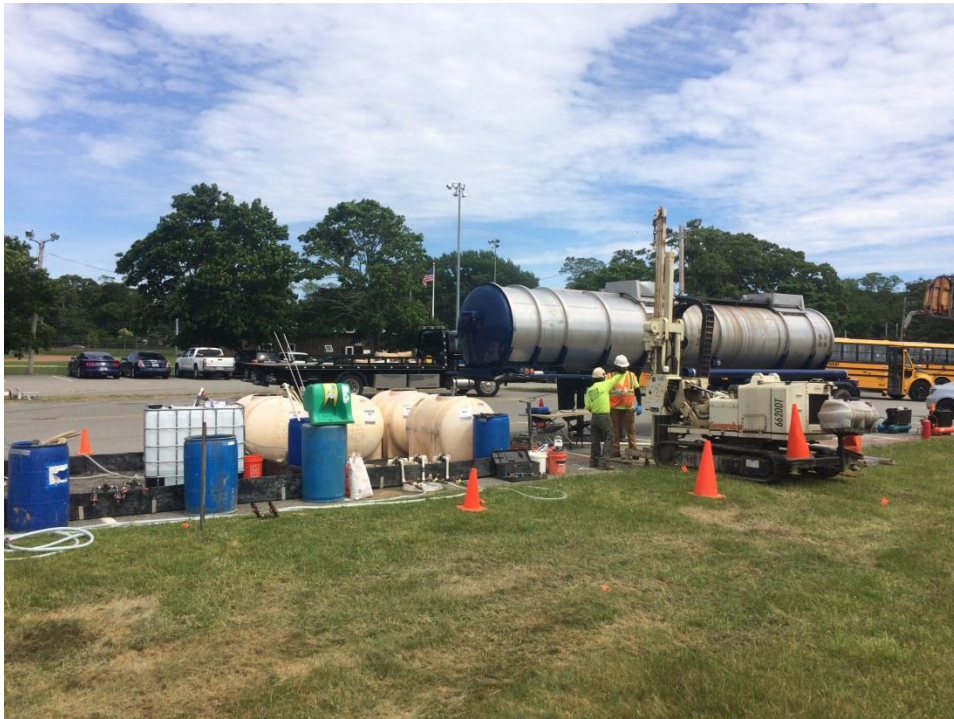
Mixing tanks for EVO.
