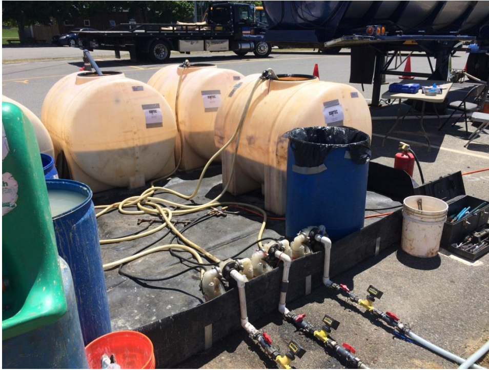
Mixing area which provides dilution for the EVO prior to injection. Pumps are shown which pumped the EVO to the direct-push points.
