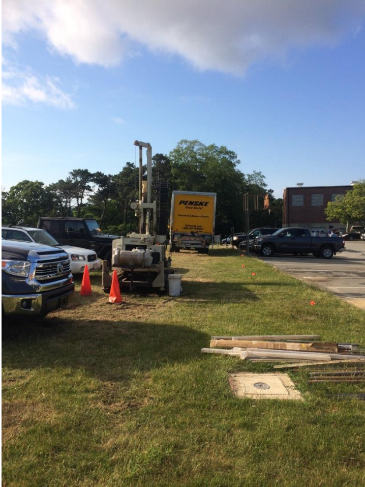
Drill rig used for direct-push points and some extra rods shown on the ground.
