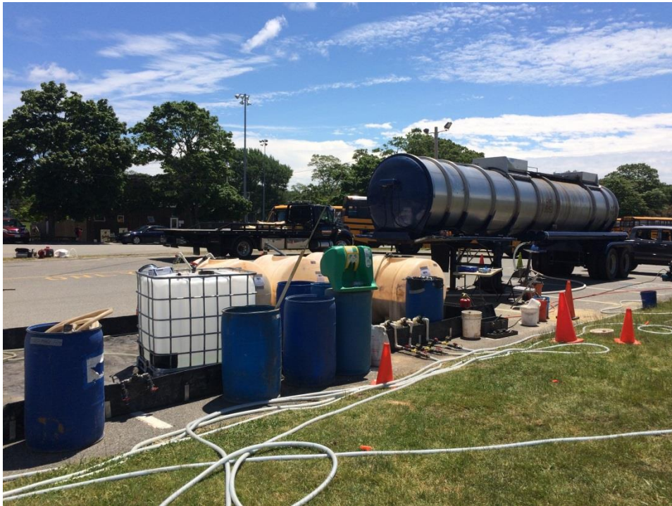
Mixing area which provides dilution for the EVO prior to injection.
