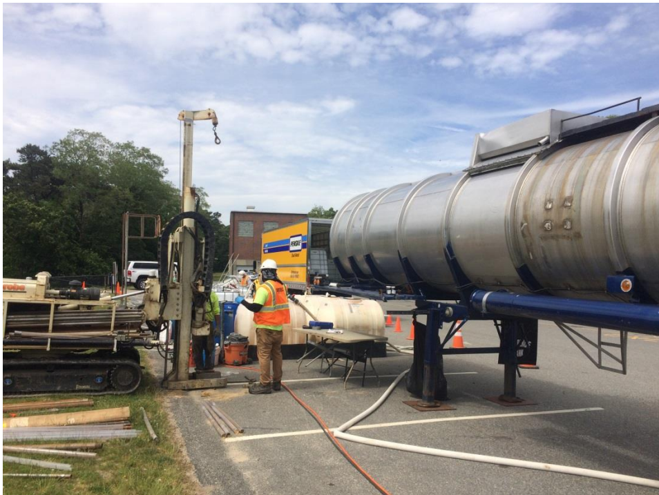
Close up of the water tank is on the right and the drill rig on the left.
