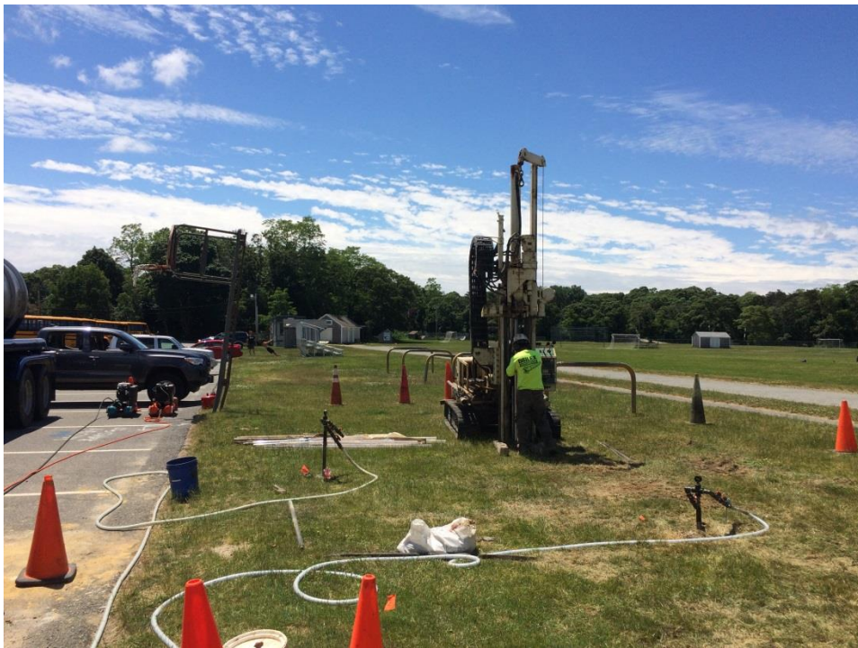
Drill rig being used for direct-push points. Two in-progress points are shown on each side.
