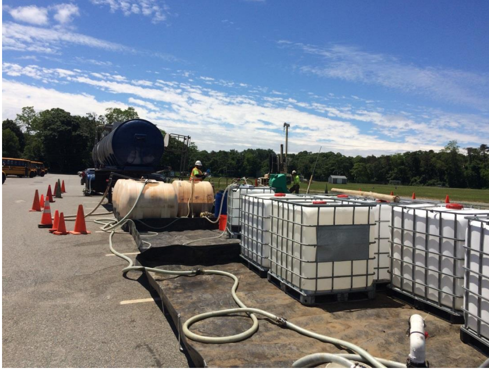
Cones on the left blocking off the water tanker and EVO mixing tanks area.
