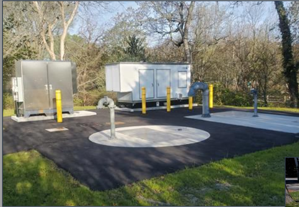
Pump Station 1 on Old Colony Way at West Rd
