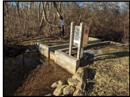
Photo 5: Pilgrim Lake outlet control structure
