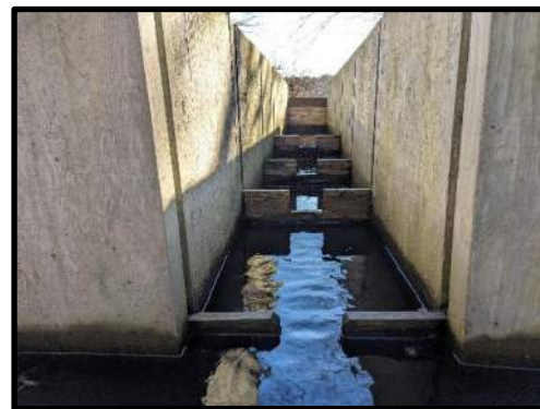
Photo 6: Pilgrim Lake outlet control structure, weir and stoplog orientation, looking south
