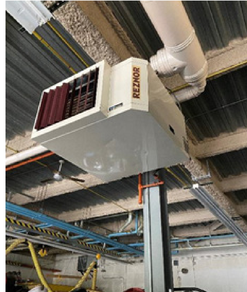
Gas Fired Unit Furnace
