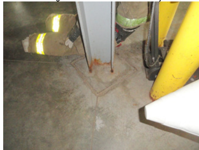
Photo #14 Basement Apparatus Room Surface rust is observed at the bottom of the steel column
