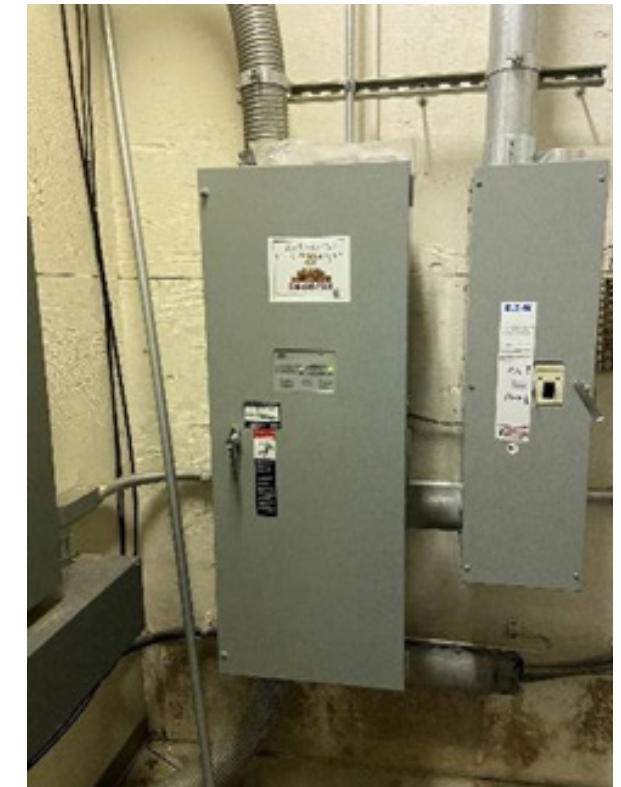
Automatic Transfer Switch
