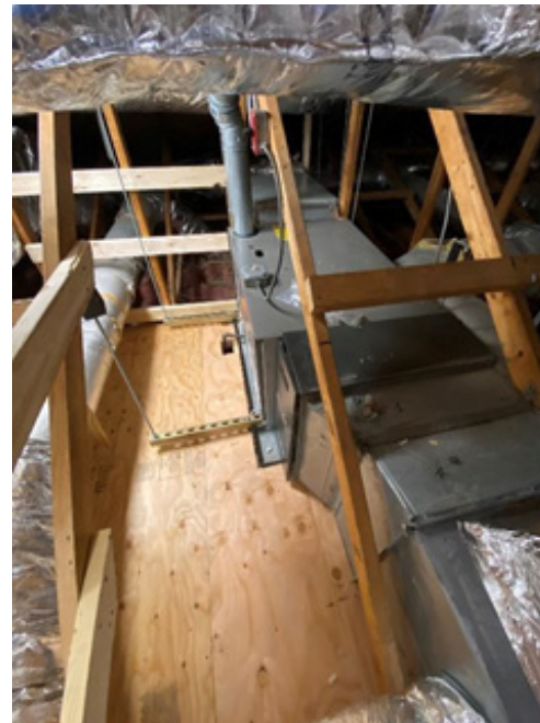
Furnace Unit in Attic Space
