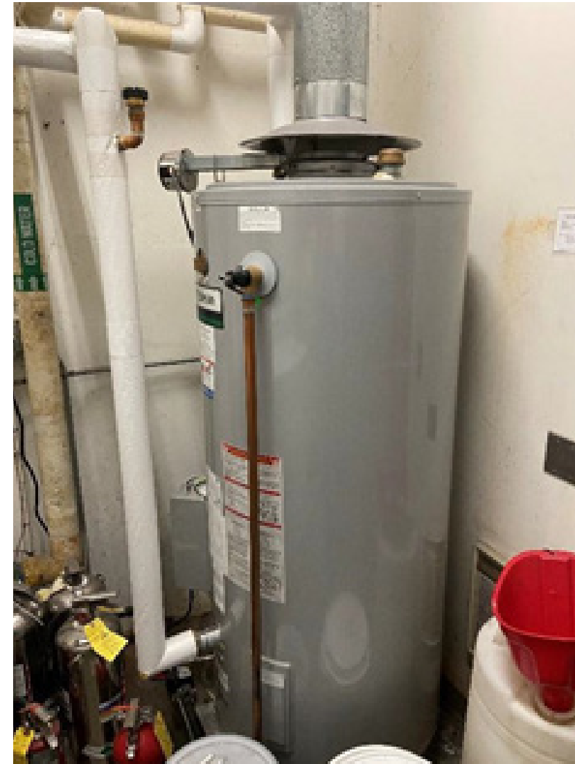
Gas Fired Water Heater
