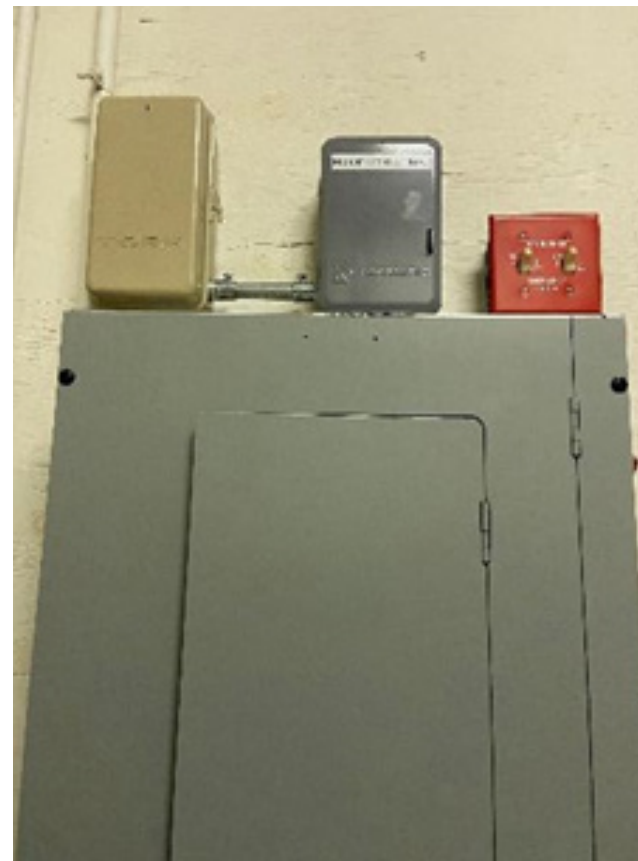
Newer Electrical Panel
