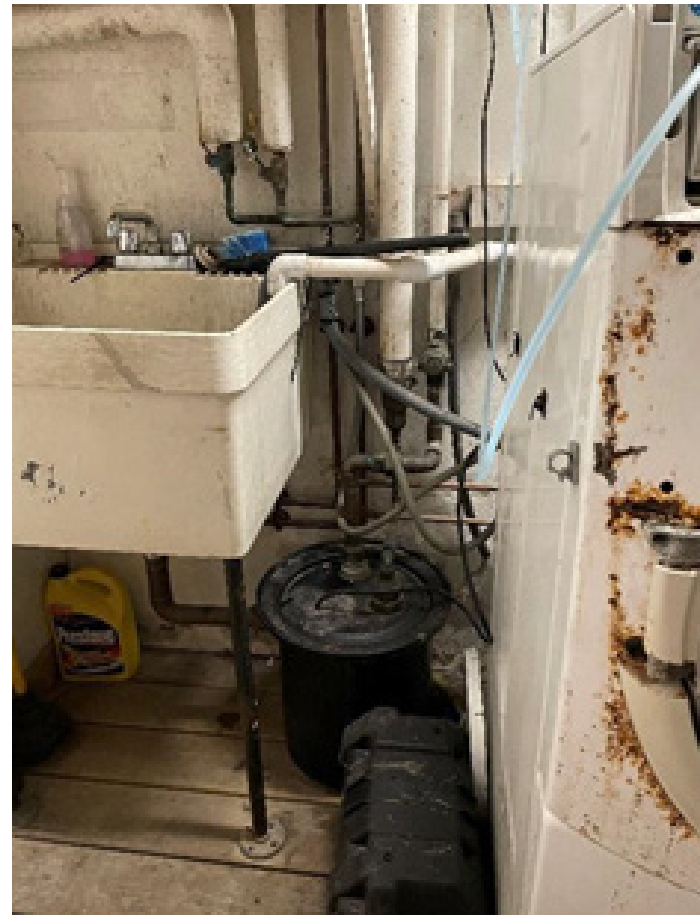
Ejector Pump for Laundry Tub
