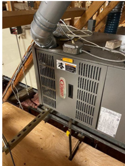
Furnace Unit in Attic Space
