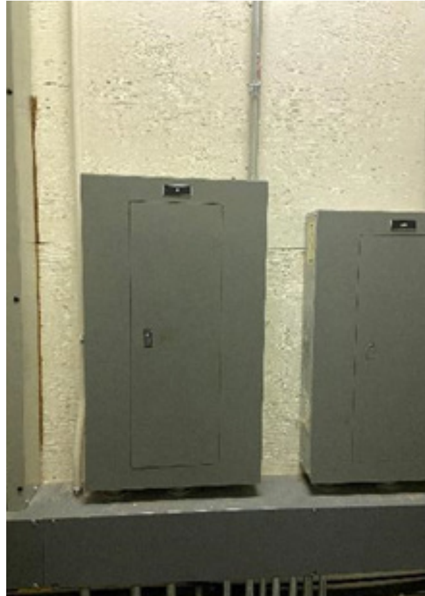
Older Electrical Panels
