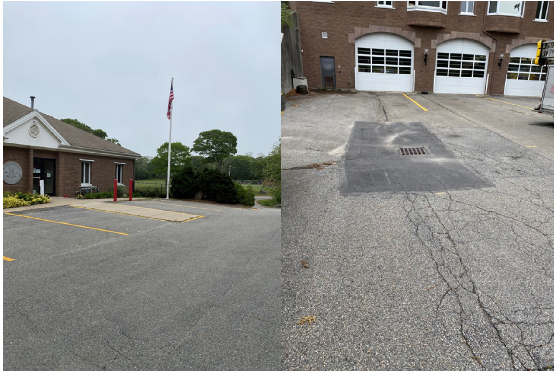
Figure 6: Existing asphalt conditions - Public entrance (left); Lower Apparatus Bays (right). Varying levels of pavement deterioration.
