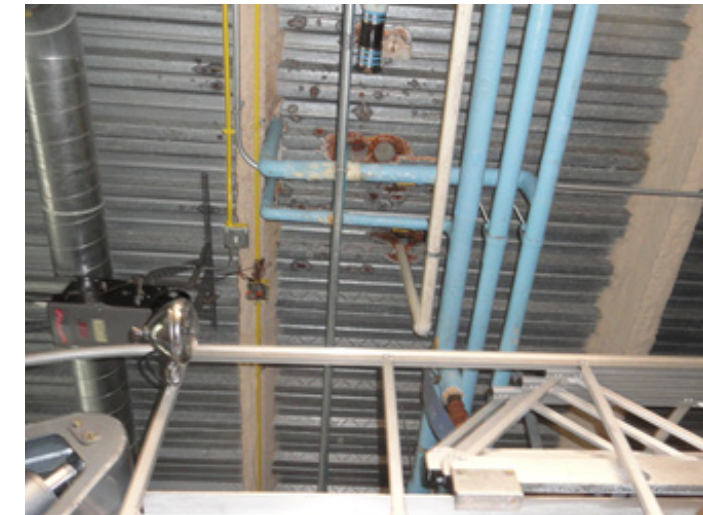
Photo #15 Underside of first floor concrete deck above the apparatus front north bay Surface rust is observed at the steel deck and floor penetrations
