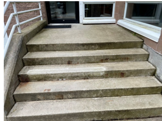
Photo #4 Building West Elevation Concrete steps with minor cracks and surface rusting observed
