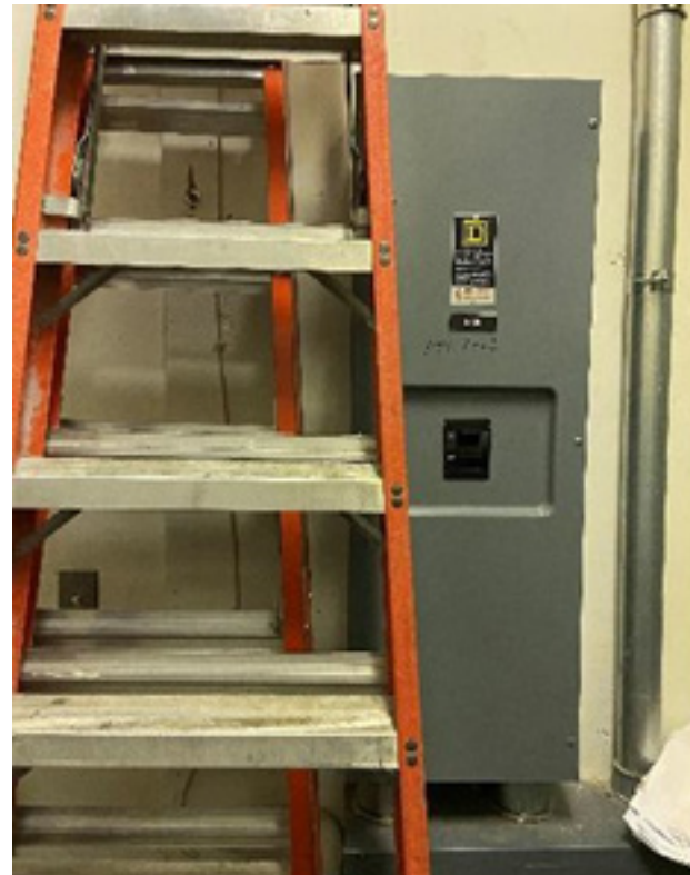
Electrical Service Equipment
