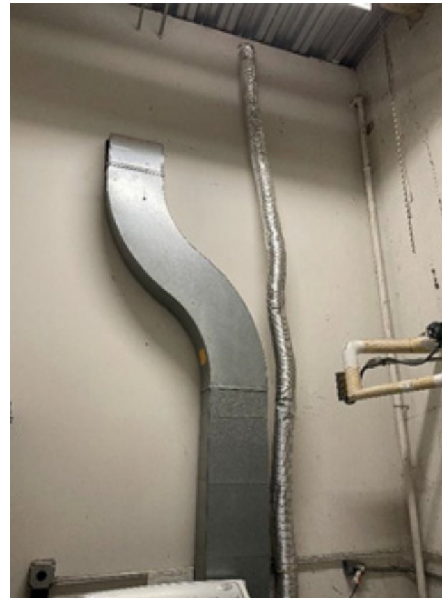
Dryer Exhaust and Relief Ductwork
