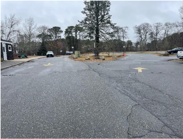
1. Pavement is patched and cracked.
