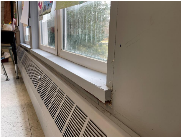
7. Windows have failed and sills water damage is evident.
