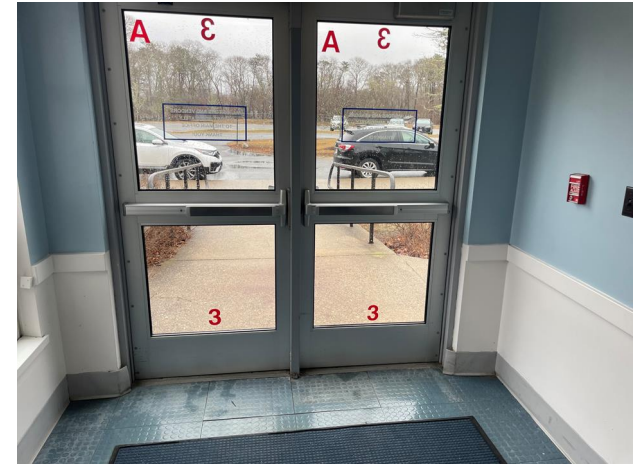
3. Rubber floors are worn.
