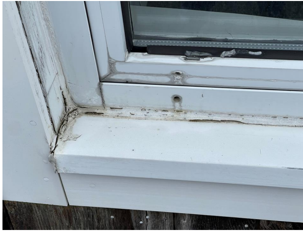
8. Sealants at windows have failed and wood trim is damaged.
