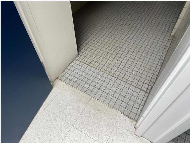
4. Ceramic Tile in Toilet Rooms is damaged.
