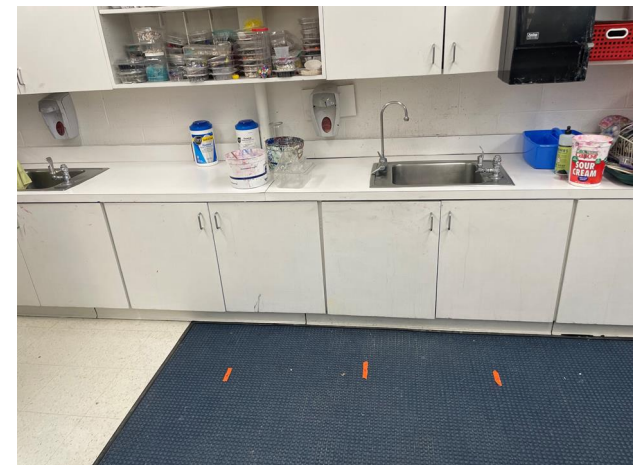
6. Sinks and drinking fountains are not accessible.
