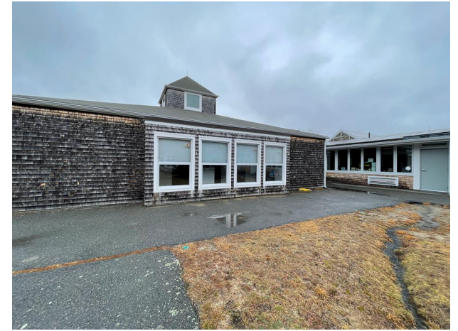
9. Drainage area has eroded soils.
