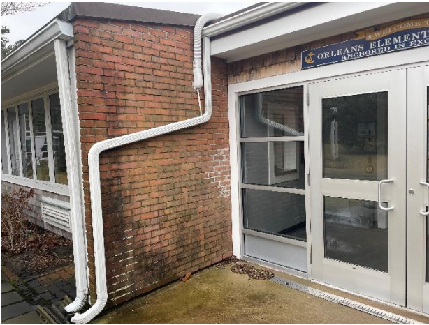
1. Brick is discolored adjacent to main entry.
