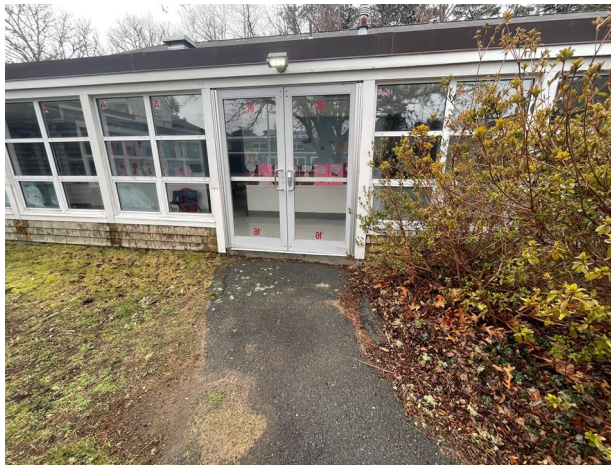
5. Shingles in some areas are too close to finish grade.
