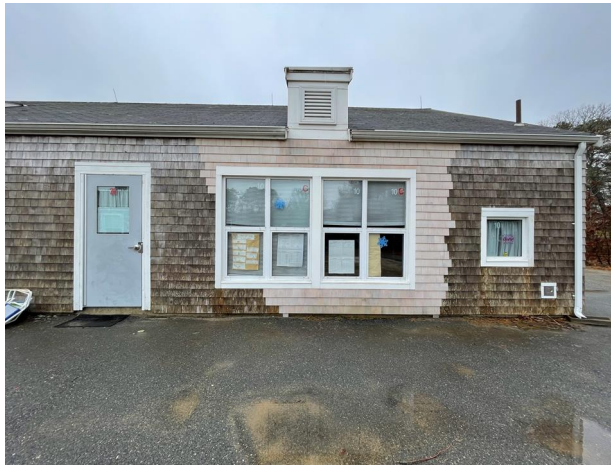
11. Indication of extent of repair required at damaged windows.
