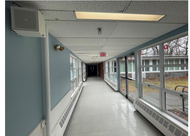
6. Fire alarm system is outdated.
