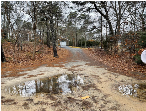
5. Teacher parking area is non-compliant and unpaved.
