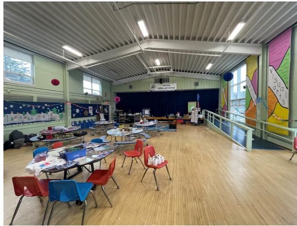
2. Lighting is outdated.
