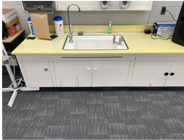
8. Classroom casework is damaged.
