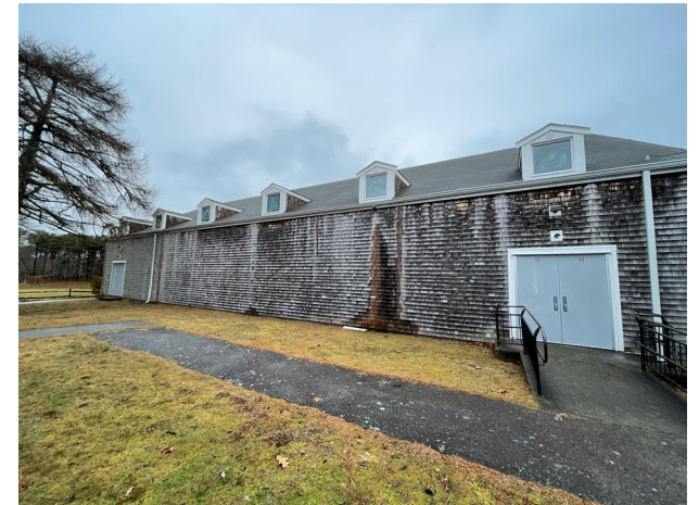
12. Eaves are lacking adequate overhang to prevent water damage.
