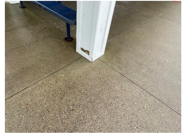
3. Column covers are water damaged.
