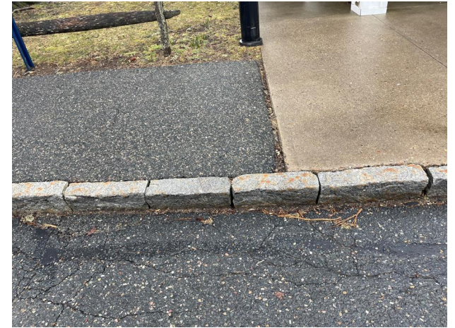
3. Deep gap between bituminous and concrete walkway.
