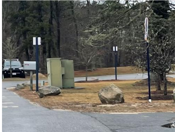
5. Site lighting is inadequate and transformer is unprotected.
