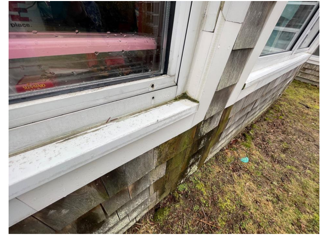
9. Damaged wall and shingles due to window failure.
