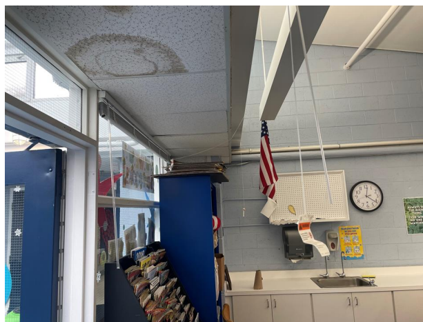
11. 2x4 Acoustic Ceiling Tiles are stained.
