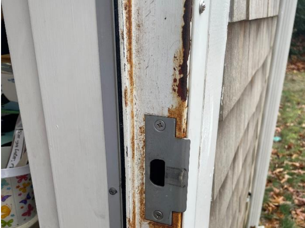
16. Door frames are rusted.
