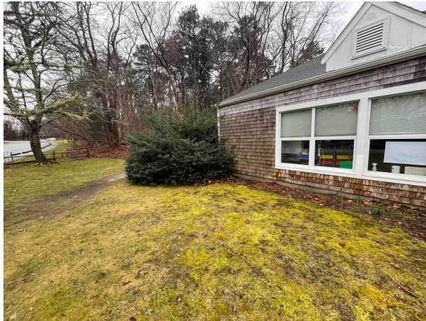
17. Wood trim is damaged.
