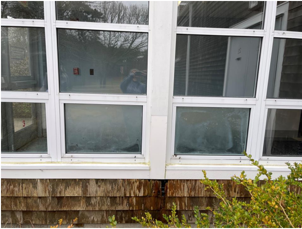
7. Many windows in 1990's addition have failed seals.
