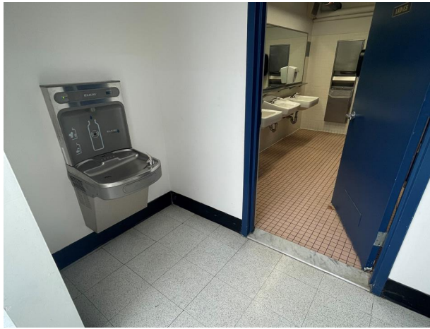
2. There is inadequate clearance at drinking fountains.
