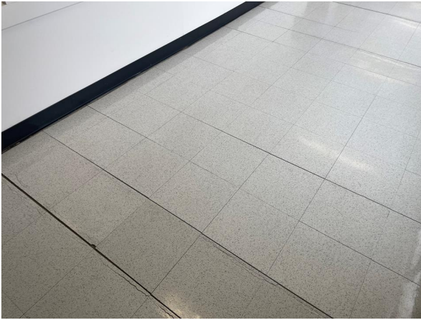
1. VCT floors are damaged.
