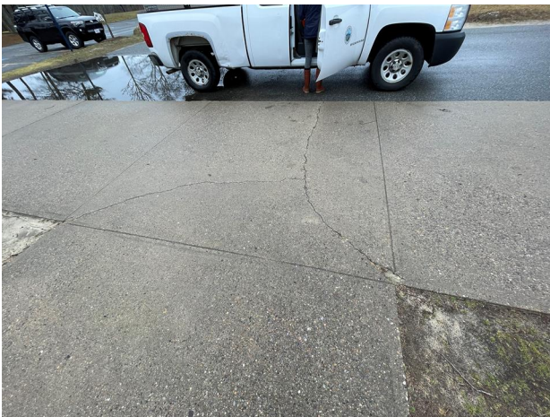
4. Concrete sidewalk is cracked.
