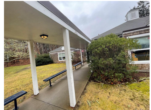
6. Soffits and wood fascia is peeling.
