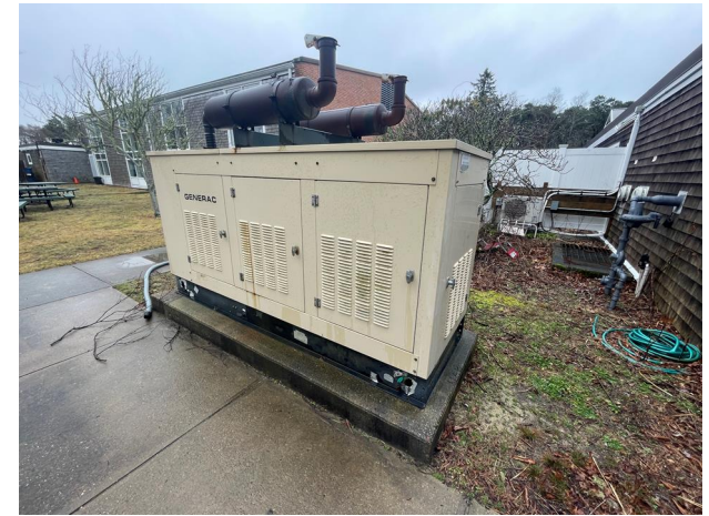
3. Generator is past its anticipated useful lifespan.
