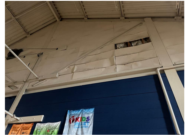
9. Metal Panels in Gym are damaged.
