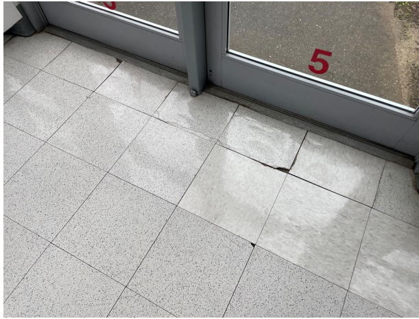
2. VCT floors are cracked and mismatched.
