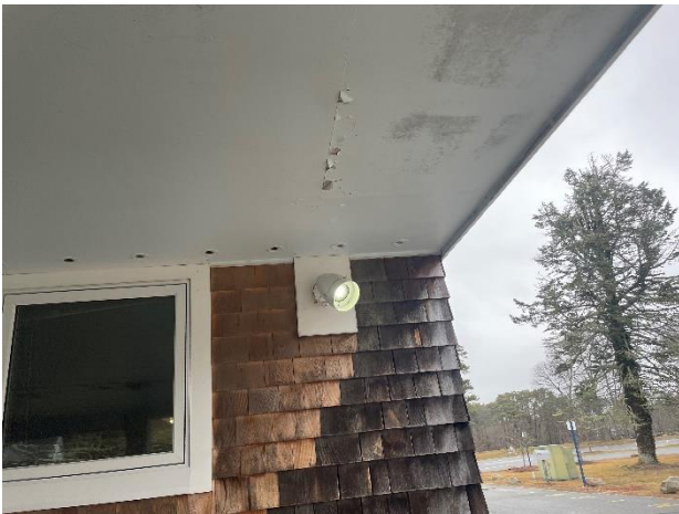
4. Paint is peeling on soffits.
