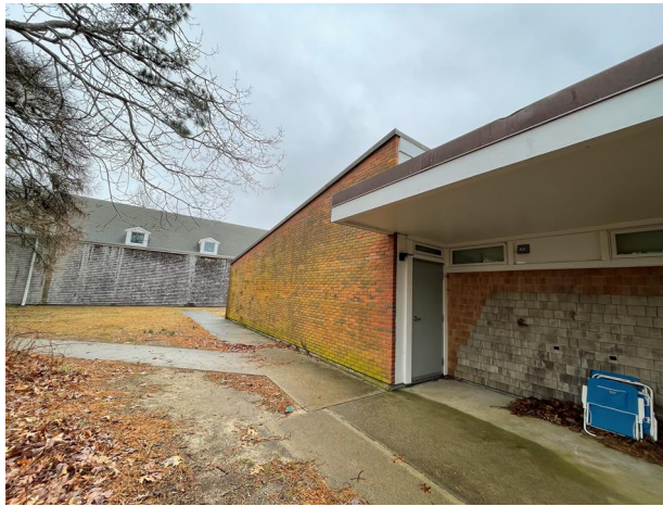
2. Brick is discolored on north elevation.
