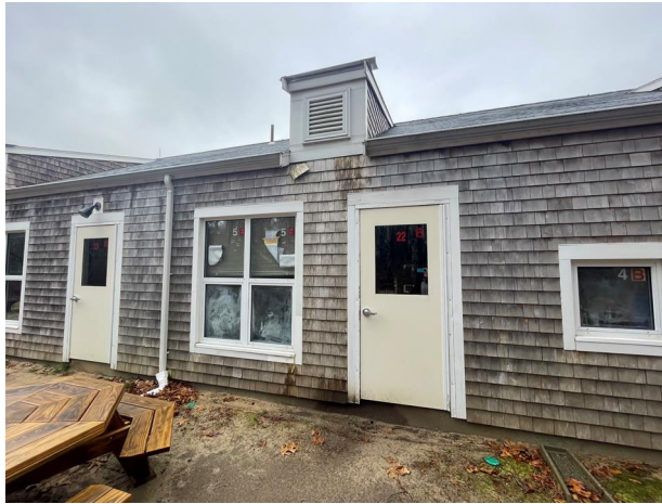
14. Water damage is evident at vent dormers.
