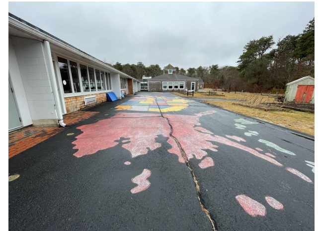
12. Bituminous play area is heavily cracked.
