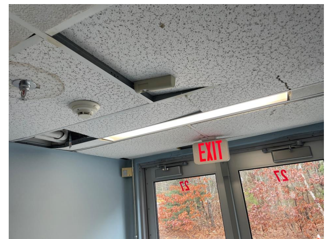
12. 2x4 Acoustic Ceiling Tiles are damaged.
