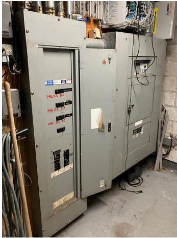
1. Electric/utility room is undersized for equipment upgrades.
