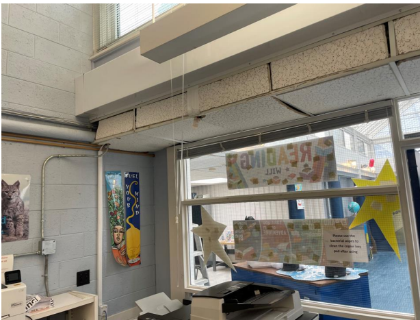
10. Acoustic Ceiling Tiles are damaged.
