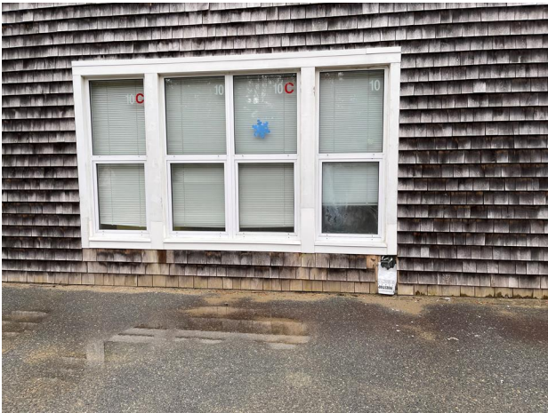
10. Window failure has caused damage to shingle siding.
