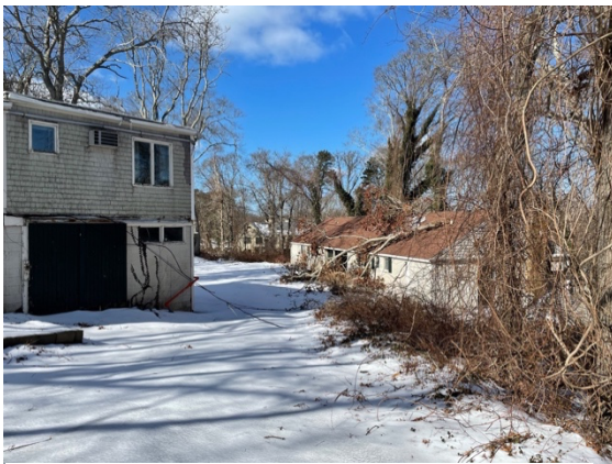
Downed tree limb, southeastern building.
