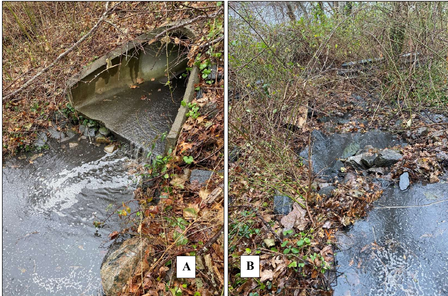
Figure IV-17. Route 28 Stormwater Runoff Pipe to Crystal Lake. A 24 inch pipe (A) collects stormwater runoff from an undetermined portion of Route 28 and discharges the runoff first to a small basin (~0.7 m 3 ) then down a ~15 m rip-rap path (B) to the lake.
