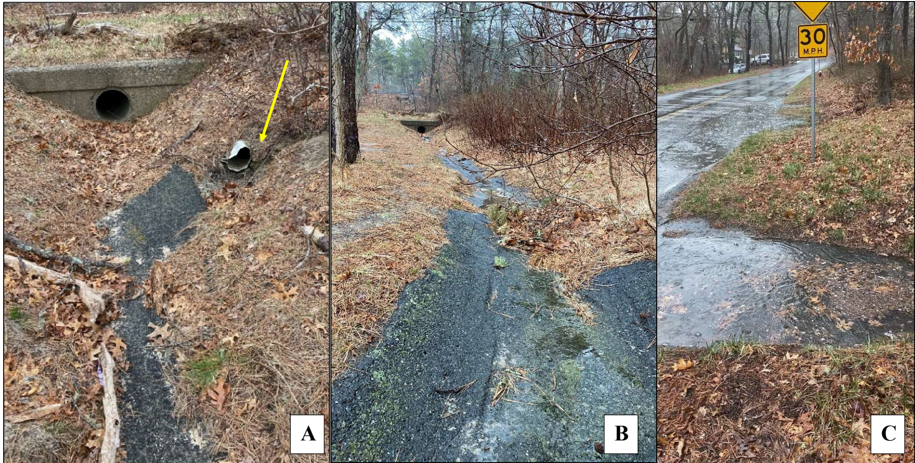
Figure IV-18. Bakers Pond Road Stormwater System Direct Runoff Discharge to Baker Pond. The partially occluded corrugated metal pipe (shown at the right in A) discharges stormwater runoff overflow from a connected series of three leaching stormdrains on the east side of Bakers Pond Road and just south of the Baker Pond town beach (stormdrains shown completely flooded on March 28, 2021 in C). The other pipe (installed in a headwall) does not discharge stormwater. When stormwater overflow occurs from the Bakers Pond Road stormdrains, it flows down the asphalt channel (shown in B) to within approximately 20 ft of the pond and flows over the beach into the pond. Stormwater monitoring conducted during the current project suggests that flow into the pond only occurs when the stormwater drains overflow and this only occurred among the three monitored storms when the precipitation rate was 0.2 inches/hour or more. Review of the locations of stormdrains along Bakers Pond Road shows that the three catch basin collect stormwater from approximately 280 m of road length.
