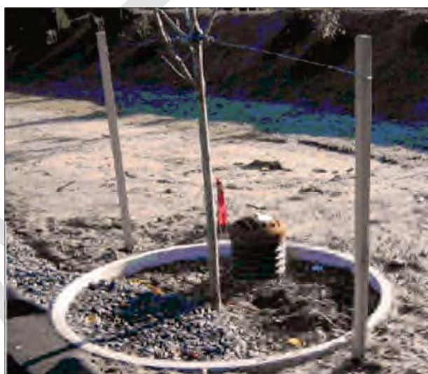
Source: Massachusetts Stormwater Handbook Figure 5-4. Newly constructed tree box filter.
