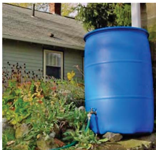
Source: Massachusetts Stormwater Handbook Figure 5-8. A 55-gallon rain barrel collecting rainwater from a residential rooftop.
