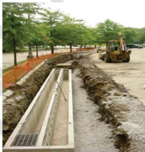
Source: Massachusetts Stormwater Handbook Figure 5-5. Sand filter system being installed at the edge of a parking lot.
