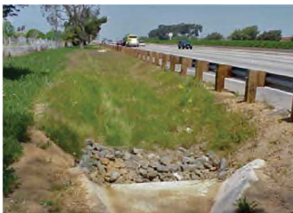
Source: Massachusetts Stormwater Handbook Figure 5-6. Grassed swale adjacent to a highway.
