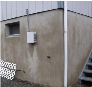
Figure 4 – Typical Exterior Control Panel
