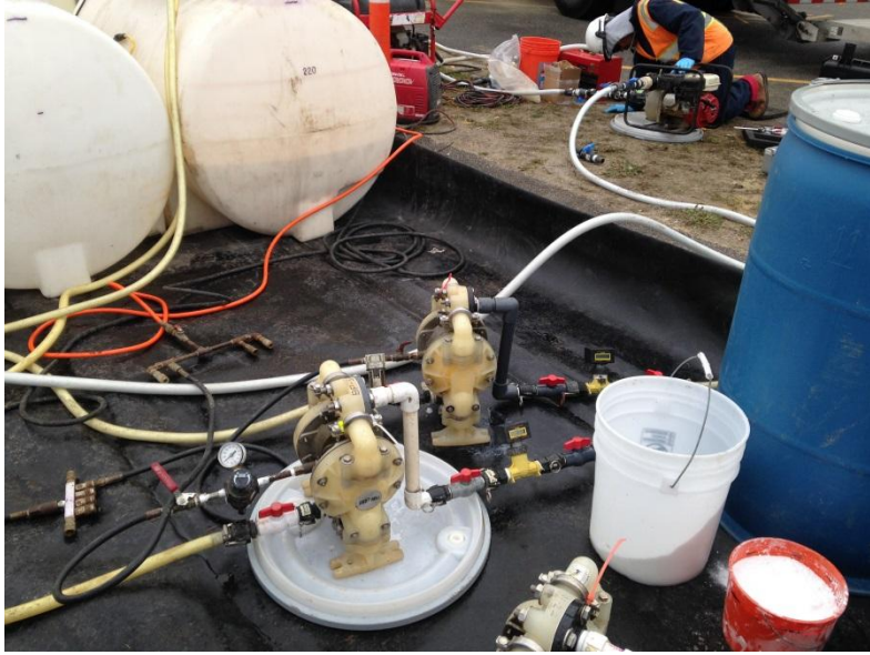
Figure 3: Injection Transfer Pumps
