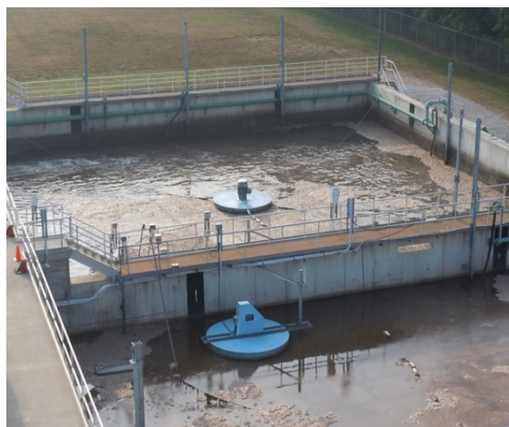
Figure 3: Sequencing Batch Reactors at Different Stages (Aqua-Aerobic Systems, Inc.)
