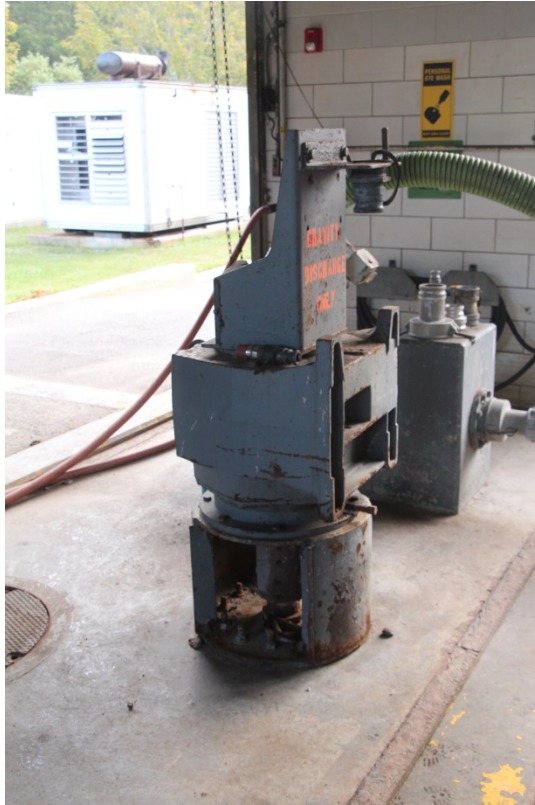
Septage Equalization Tank Mixer
