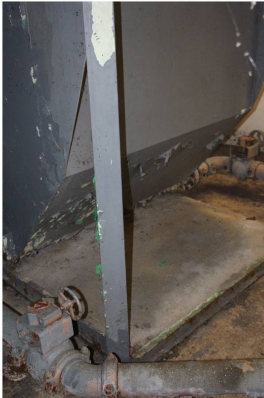
Lamella Clarifier Corrosion
