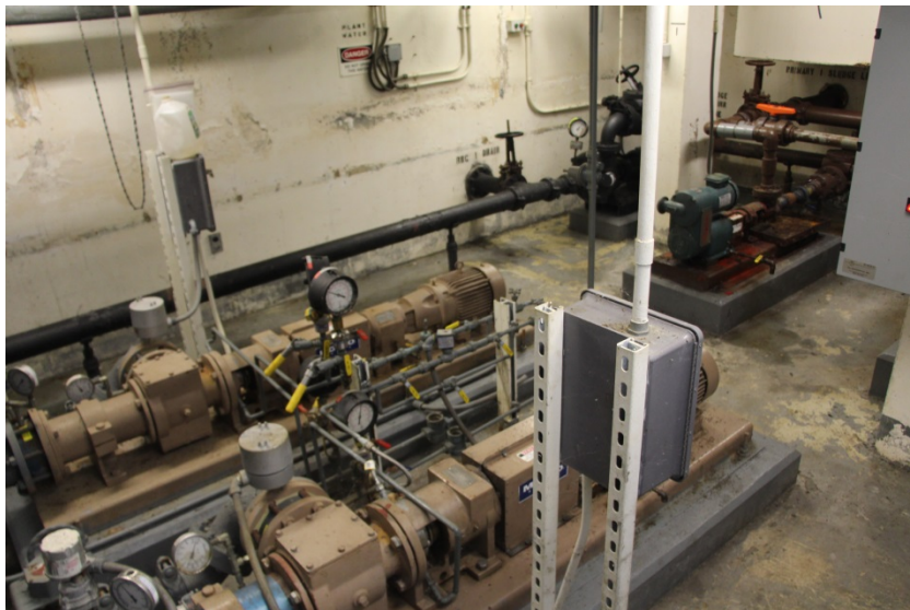
Intermediate Pumps Requiring Rebuild
