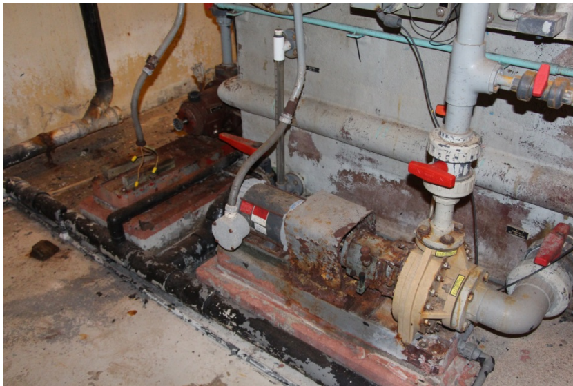
Main Odor Control Wet Scrubber Recirc Pump
