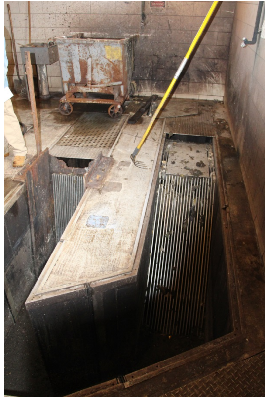
Severe Corrosion on Receiving Area Screen
