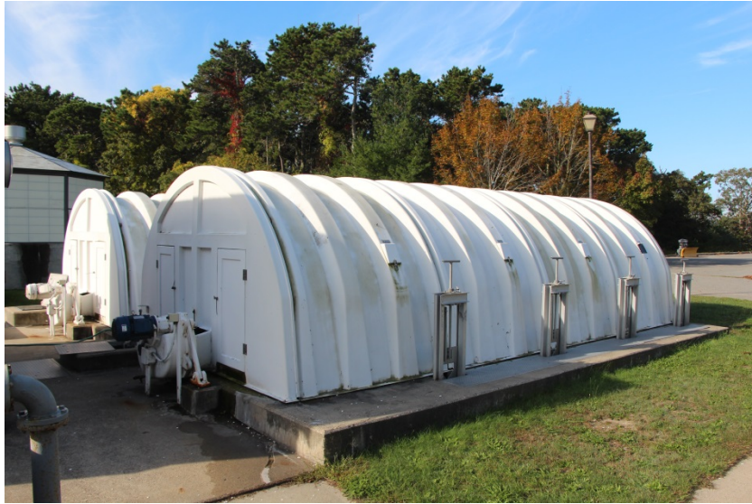
Four RBCs in Total – Two Original and at End of Life
