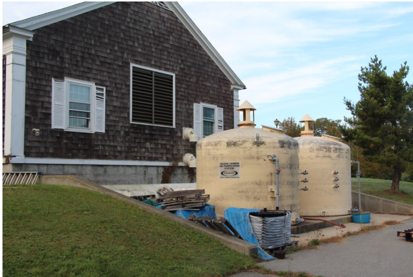
Main Odor Control Carbon Canisters
