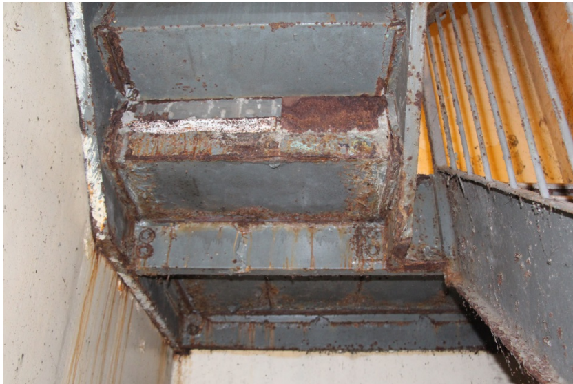
Severe Corrosion in Grit Wetwell Staircase
