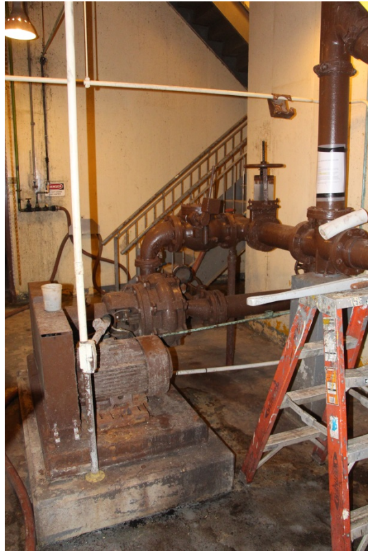
Grit Feed Pump – Corrosion and Abrasion Issues
