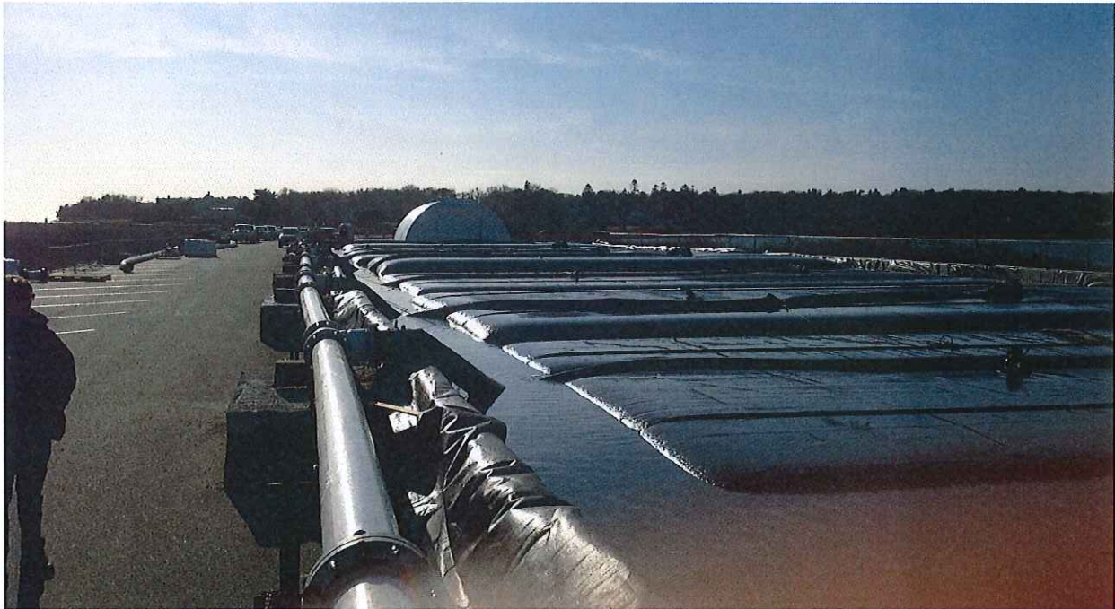
Geotubes, collection manifold and process building in background
