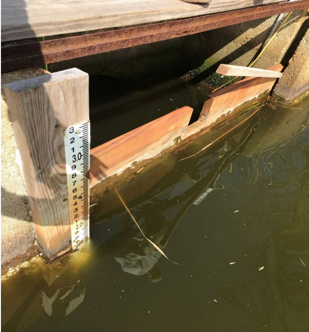
Figure II-1. Notched Board at Cedar Pond Outlet. After reviewing 2018 water levels at the outlet, Town, MassDMF, and CSP/SMASST staff agreed that the boards at the outlet could have a notch in the upper board to facilitate fish passage while also trying to limit the volume of high tides reaching Cedar Pond. Subsequent water level monitoring in 2019 showed that once a notch was added, salinity levels increased at the same rate as in 2018 when the boards were lowered. 2020 monitoring suggested that the elevation of the bottom of the notch could be increased while also attaining similar frequency of acceptable water levels meeting the Fishway Plan goals. Notch elevations are adjusted according to Fishway Plan goals for 6 inches of water over the notch bottom in the spring for spawning herring immigration (March 15 to June 30) and 2 inches of water over the notch bottom in mid/late summer to allow young of the year emigration (July 1 to November 15). No herring had been observed during more than 81 visits from 2018 through 2021, but use of fyke nets by Town and MassDMF in March/April 2022 trapped and released 30 alewife herring. Herring in the Cedar Pond Creek is one indication of improving water quality conditions in Cedar Pond.
